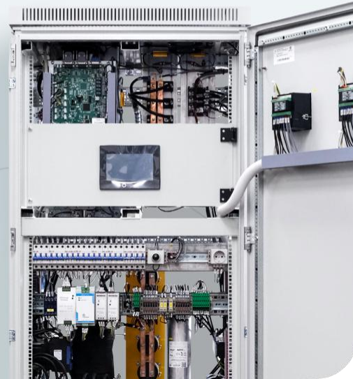
UNINTERRUPTIBLE POWER SUPPLY UNITS
