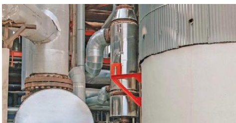
Modernization of methanol production
